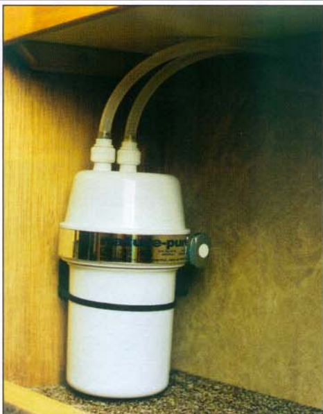
The original mounting bracket needed the assistance of a cable tie.
