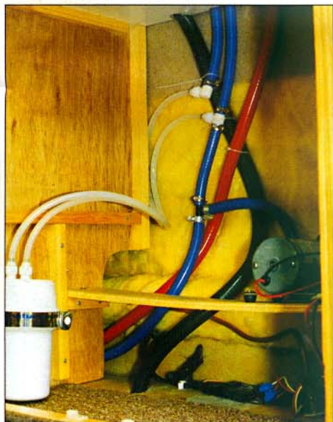
Hose layout under sink. Tee-piece is fitted into main cold water supply. Elbow mates feed from filter, to blue pipe (top left) into single faucet.
